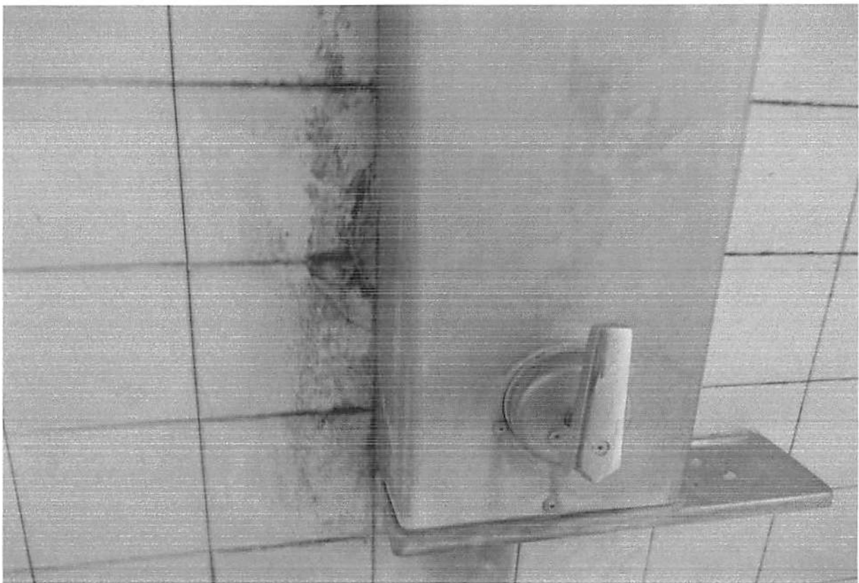
Photograph #14 Broken tiles
