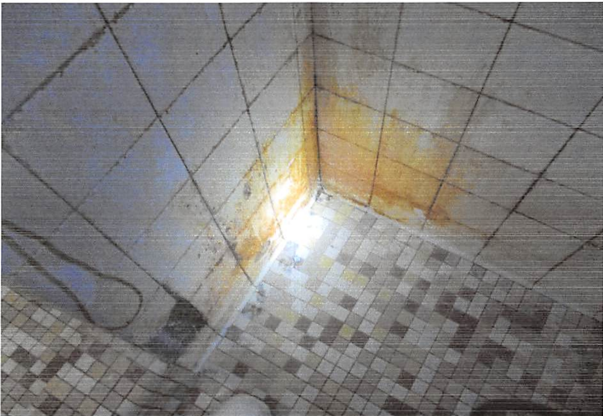
Photograph #16 Discoloration and missing tile
